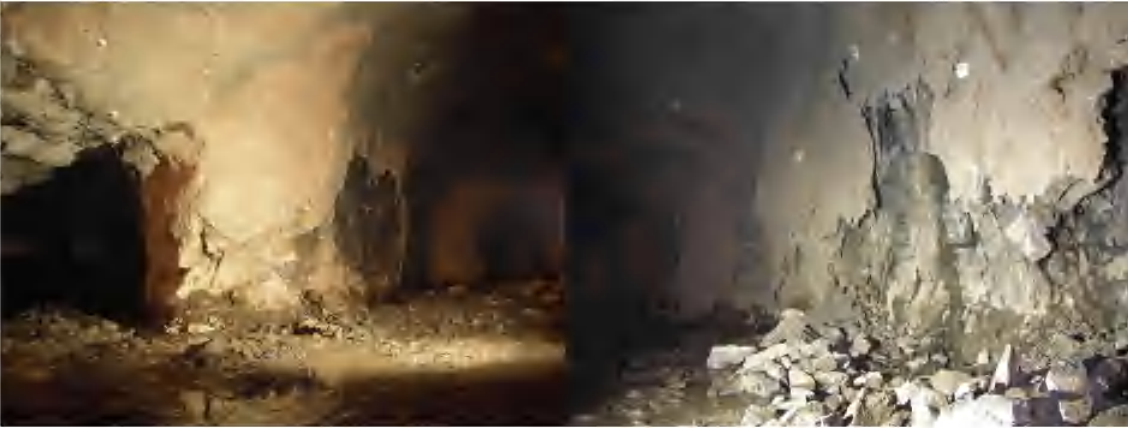
Figure 20. Spalling in the distributor tunnels
