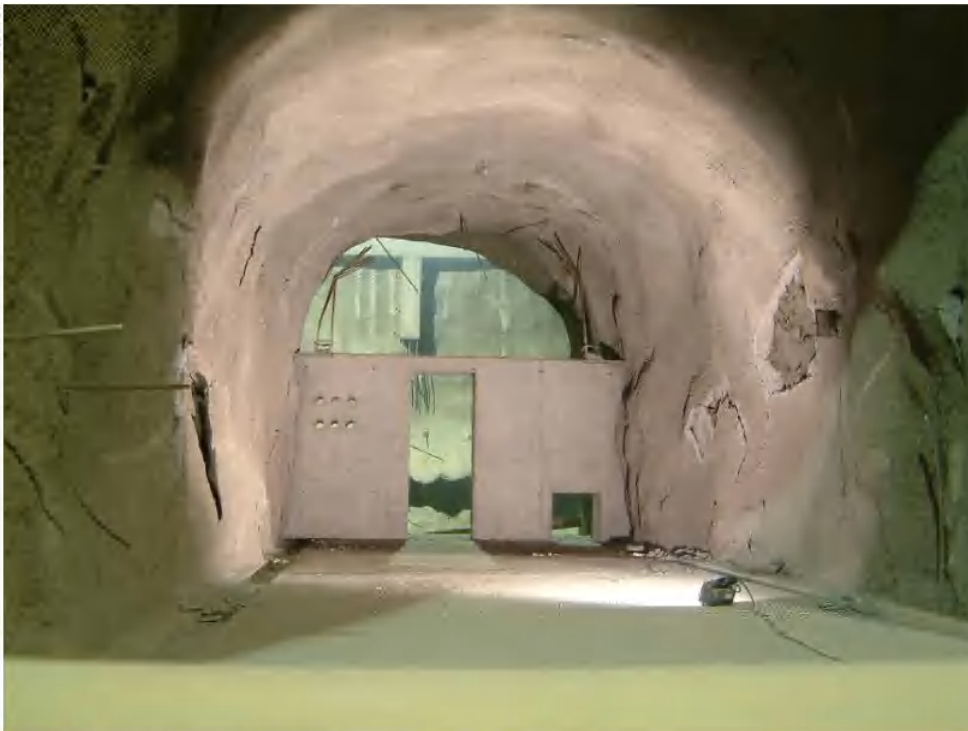
Figure 19. Spalling in the busduct tunnels
