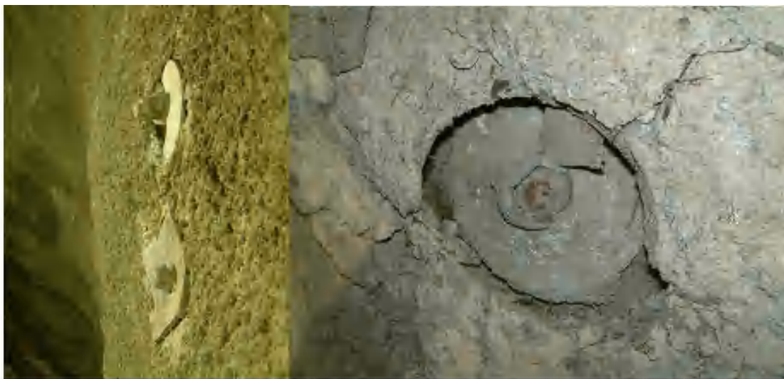
Figure 21. Bent bolt plates and nut pushed through the spherical ring
