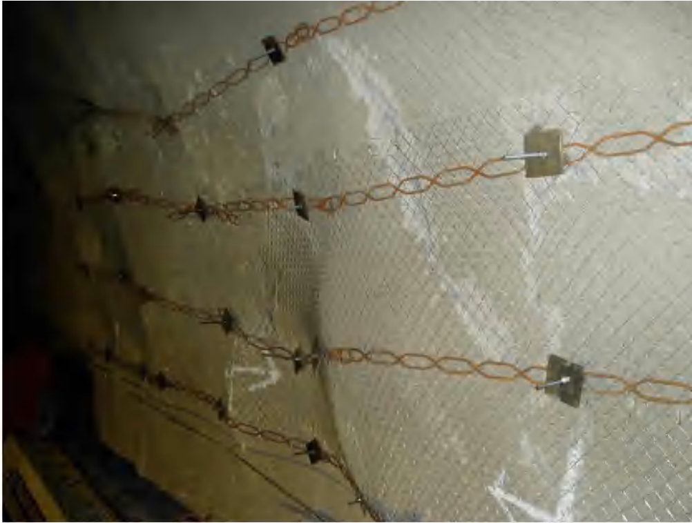
Figure 22. Chainlink mesh on the spalling area above the crane beam in powerhouse
